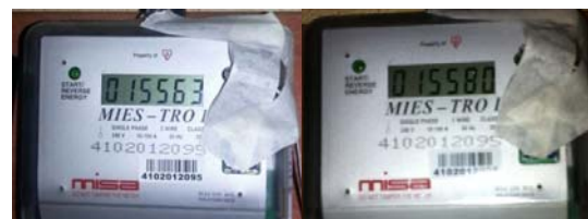
Figure 11. Electricity Meter Reading during test
