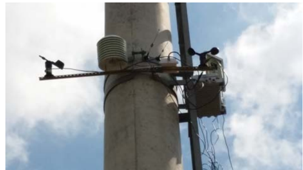
Fig.6 Device installation site
